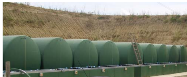
MAD leachate storage cisterns
